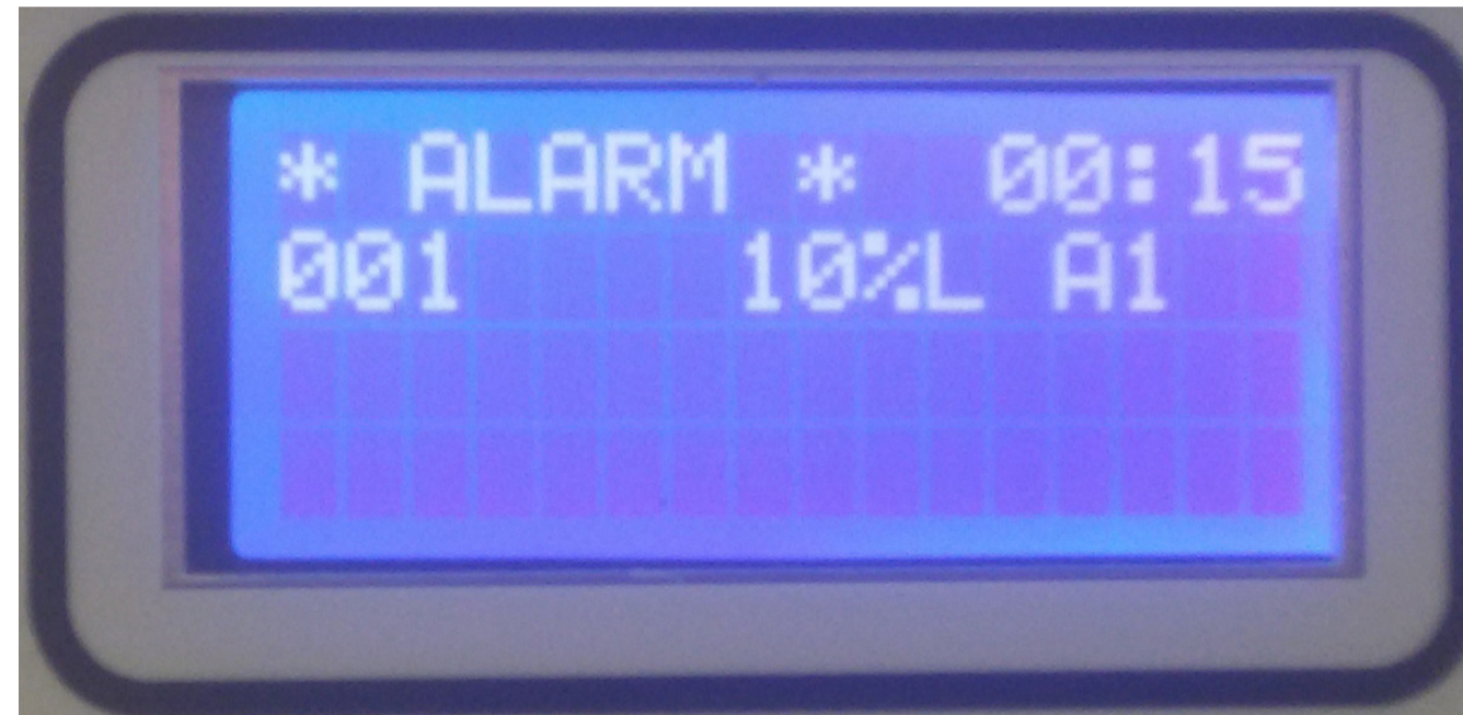
Figure 25 Typical ALARM state screen.
