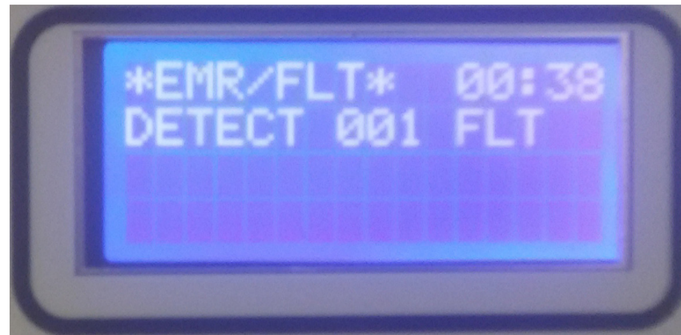
Figure 27 Typical FAULT state screen.
