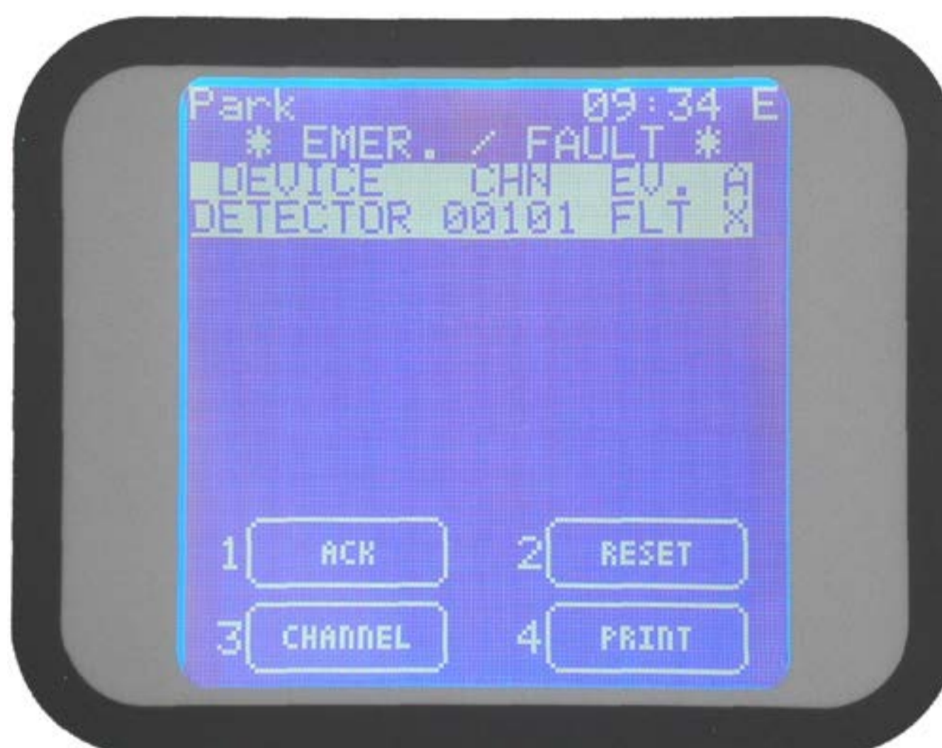
Figure 22 Typical FAULT state of the ACTIVE EVENTS screen.
