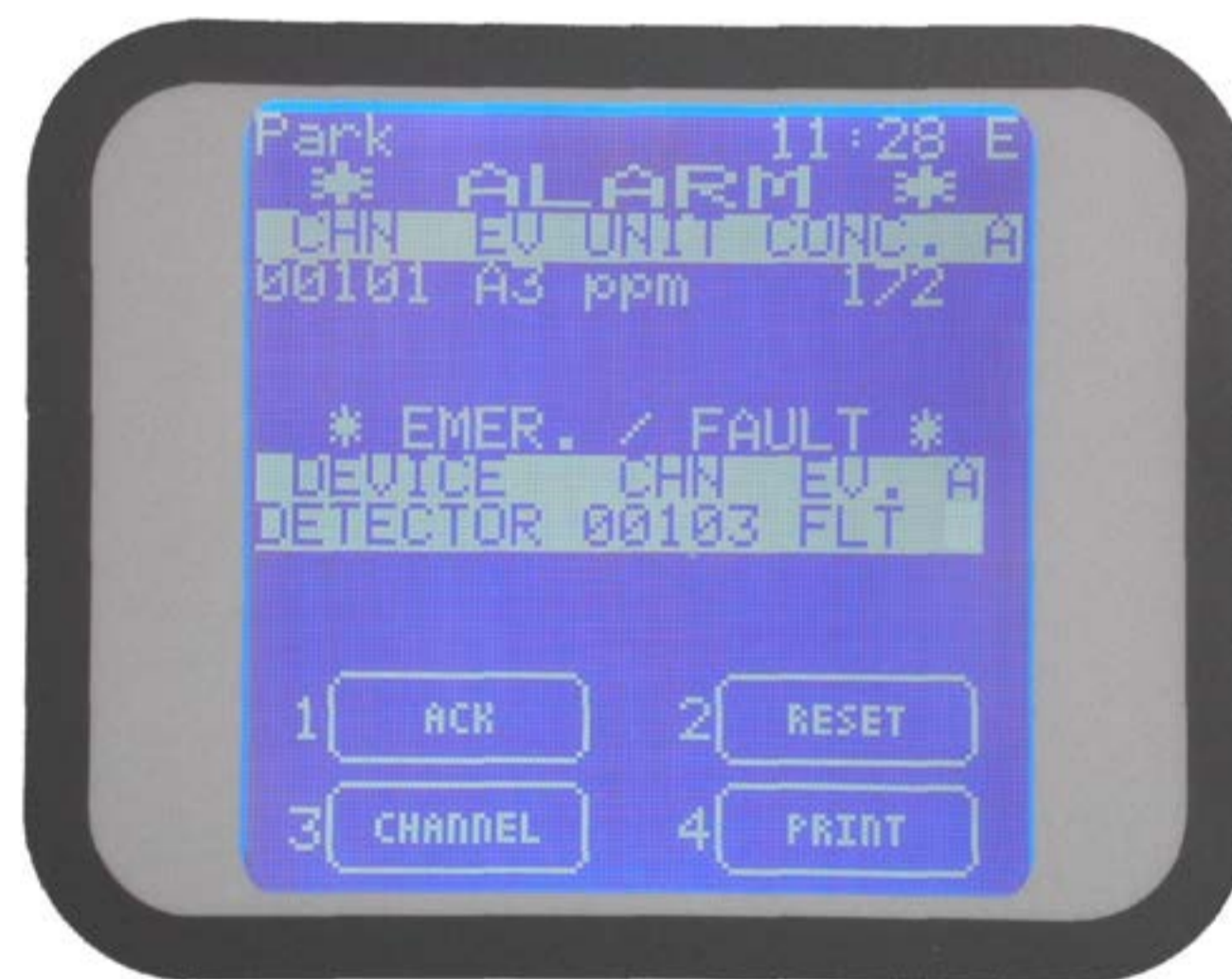
Figure 25 Active Events screen with Alarm and Fault
